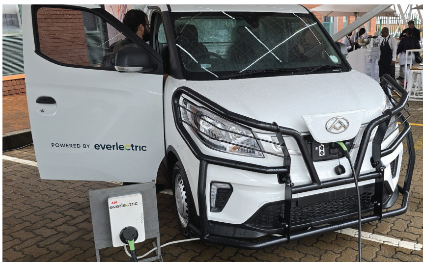
▲ UPD has expanded its renewable energy infrastructure adding 1 170 additional solar panels and several high-speed chargers.
